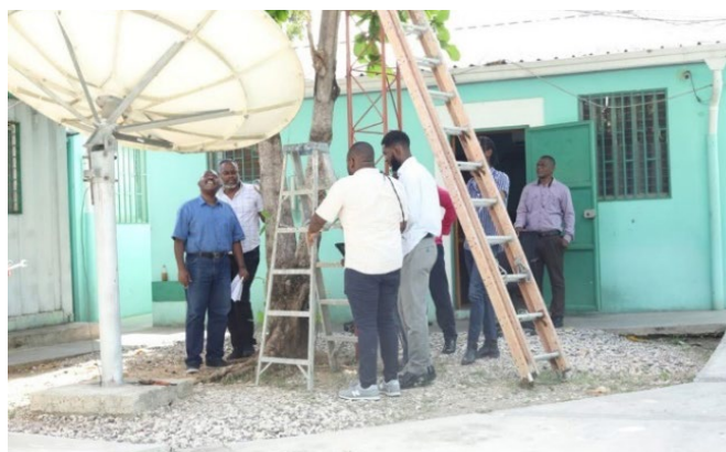
Figure 23. Enhancing data access: GEONETCast system installation in Haiti
